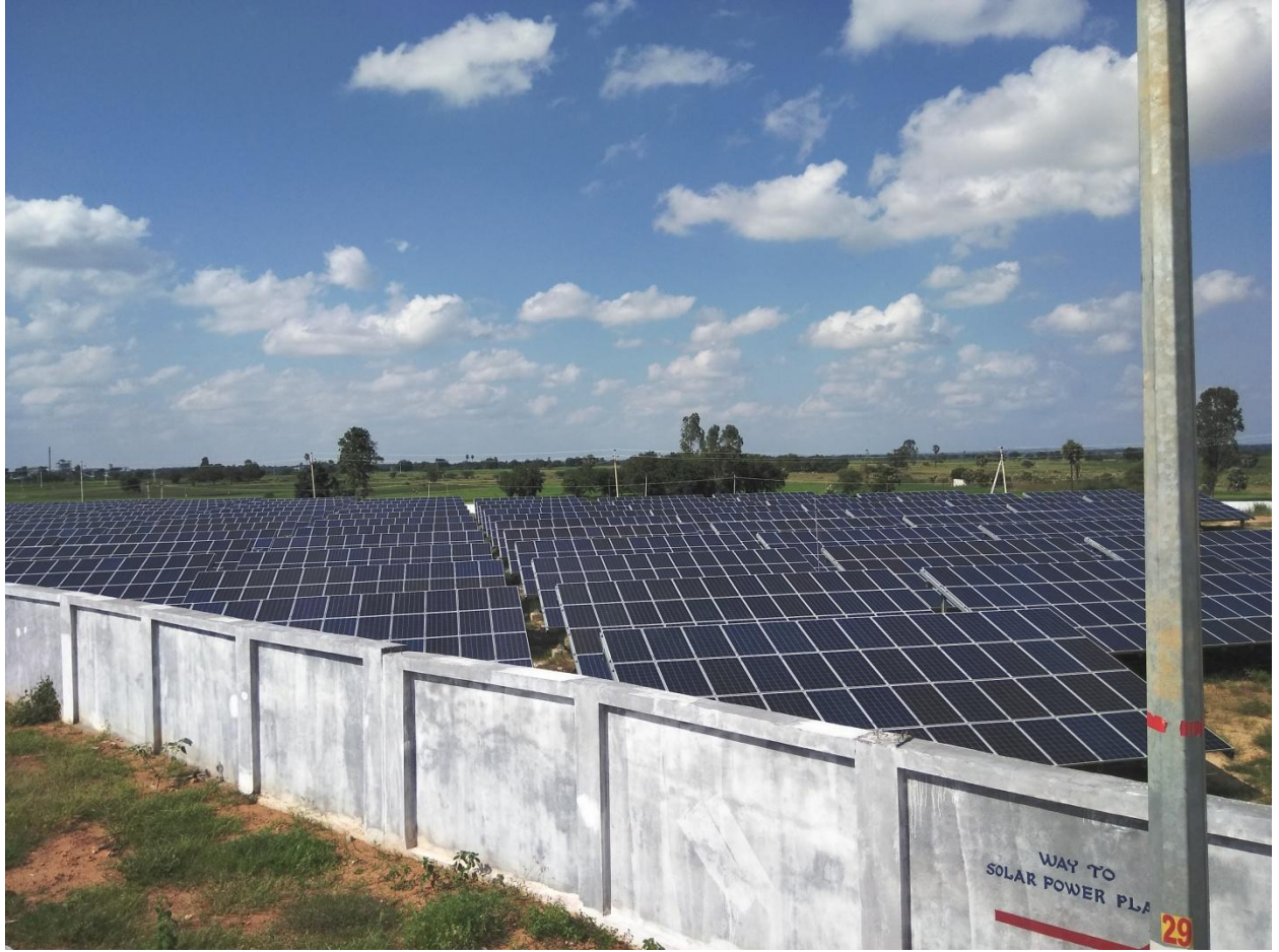
A view of Solar Panels
